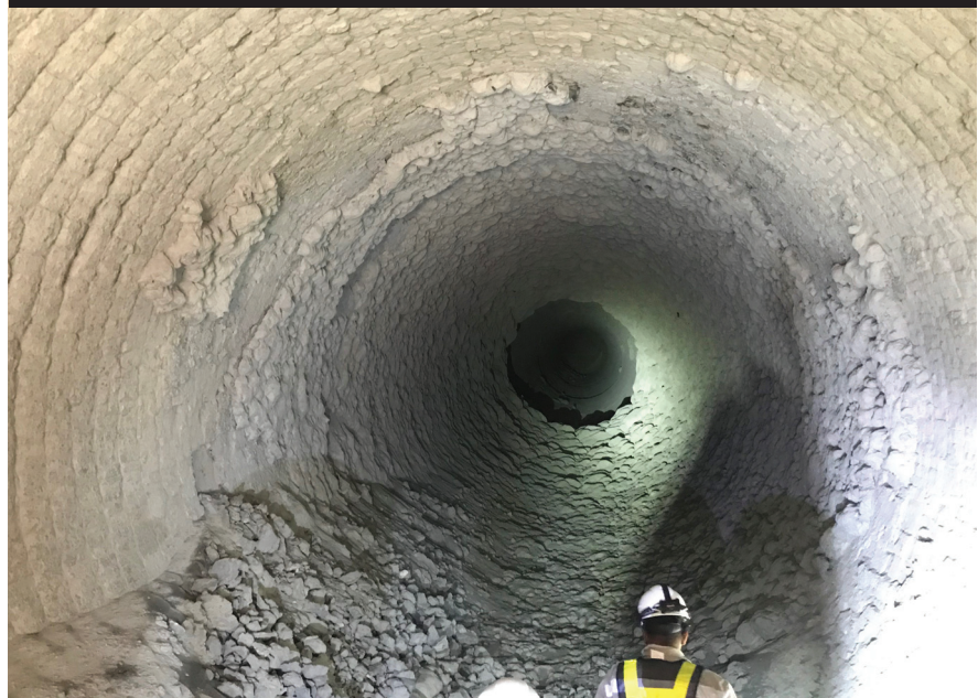
Figure 1: MultiMag performance after 704 days of continuous operation in an 4500tpd cement kiln in Thailand (photo taken in November 2019 before brick removal)
